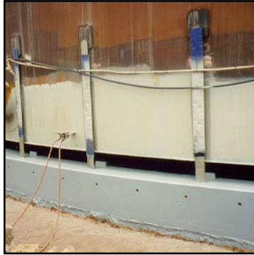
Preparation of tank and base underway. Tank jacked up and ready to install new timber
