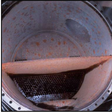
The corroded water box.
